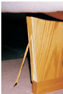
Avoid: veneer edge banded pew supports. This method is susceptible to peeling.
