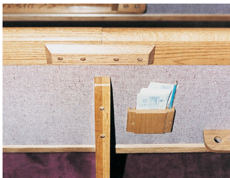
Avoid: crude brace for butt joint cap rail.
